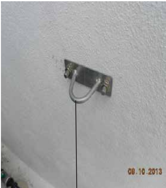
Safety hook – provided at rainwater harvest tank
